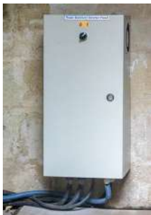
Inventor & electrical panels for water recovery system
