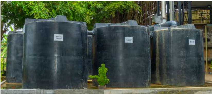
Blow Down Water Recovery System
