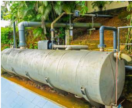
Filter Backwash Water Recovery System
