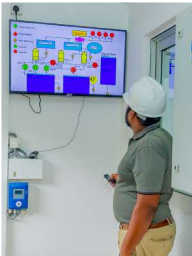
Water Treatment System Automation
