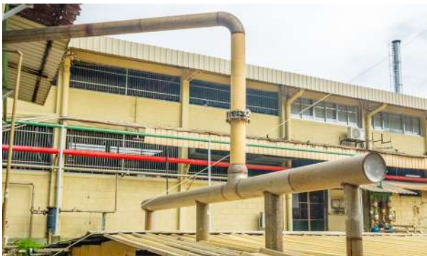
Cooling water recovery project
