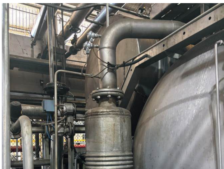
Condensate Water Recovery Project
