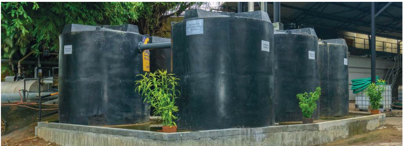
Blow down water recovery system
