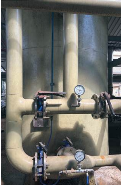
Water treatment optimization of Sand Filtration
